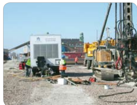
Malmö Citytunnel – Sweden Ground water screening during the construction of the City Tunnel.
