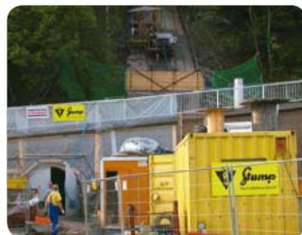
Ohra Dam, Oberhof – Germany Drilling of grout holes at the Ohra Dam.
