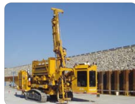
Wolf Creek Dam, Kentucky – USA Installation of grout curtain to prevent seepage.
